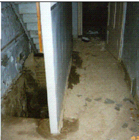
Pic 1-1 Damage inside the building
