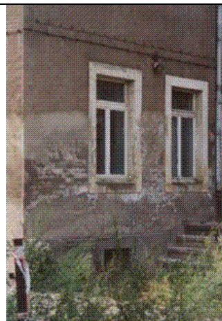
Pic 1-2 External damage to the house
